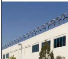
A series of small-scale roof-mounted turbines
